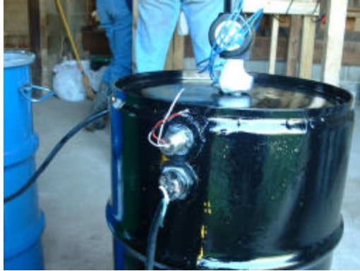
Figure 3.1.1 Heating element as seen from outside of tank
