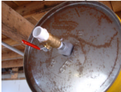
Figure 3.1.3 Heating tank fitting as seen from bottom of tank
